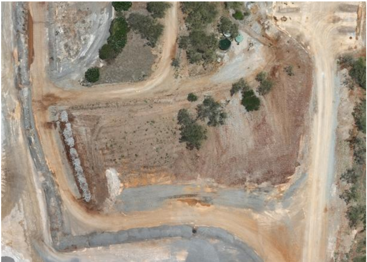
Figure 13. Pit 1 (upper) was fully backfilled in 2024 (lower) with well compacted blasted rocks and fines.
