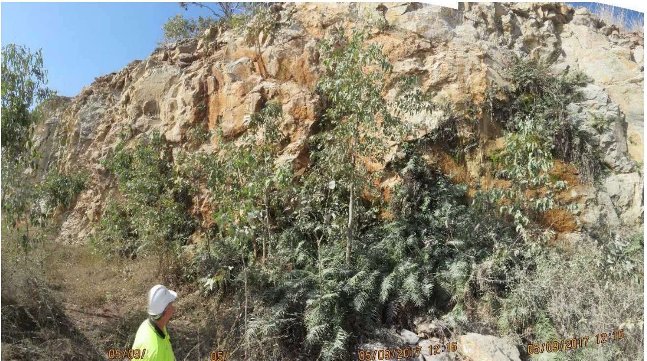
Figure 17. Water can seep from the batter of the upper bench on the east wall of Pit 4 when the level of water in Awoonga Dam exceeds \approx 40 mRL.
