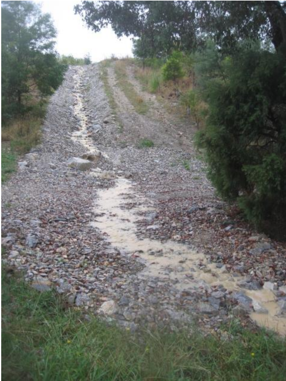
Figure 20. Example of a shallow rock lined v-drain constructed down a slope comprising erodible soil to prevent gully erosion. Similar drains will be required in sections of final upper benches comprising soil filled karst.
