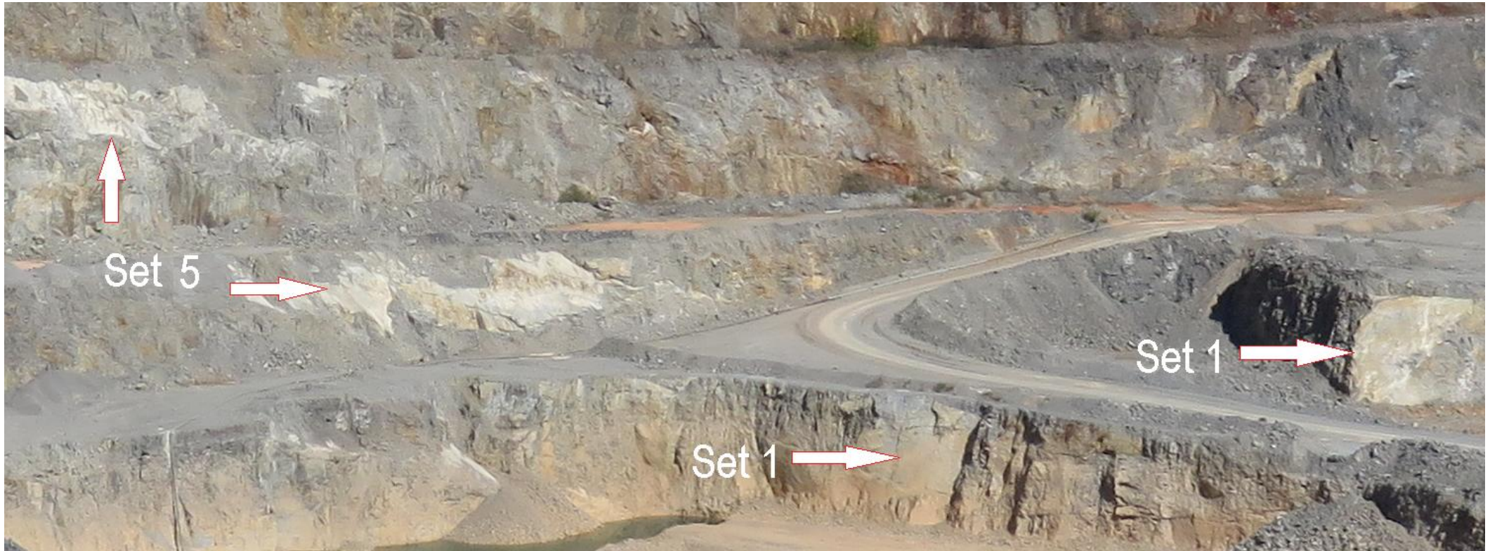
Figure 9. Examples of planar sliding on the west wall of Pit 4 involving bench scale masses of rocks sliding along bedding/cleavage from Set 1 and joints from Set 5.
